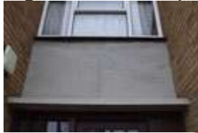
Fig 2 Asbestos panel on an external wall
