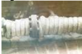
Fig 1 Asbestos insulation on a pipe
