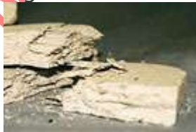
Fig 4 Pieces of Asbestos Insulating Board
